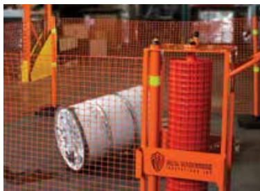
SECURE A TEMPORARY HAZARDOUS AREA
